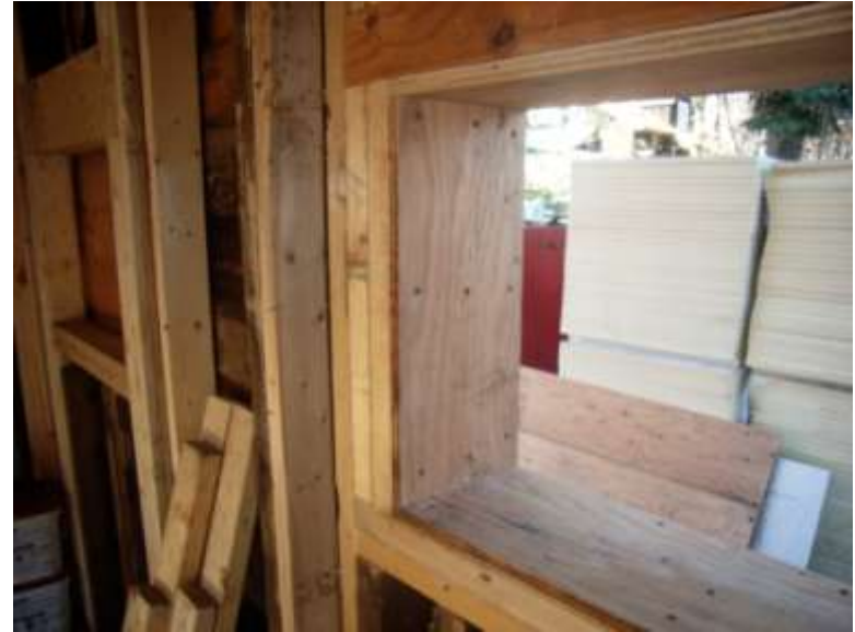
Plywood window bucks go in. (Lifts of polyiso stack in the driveway outside ...)
